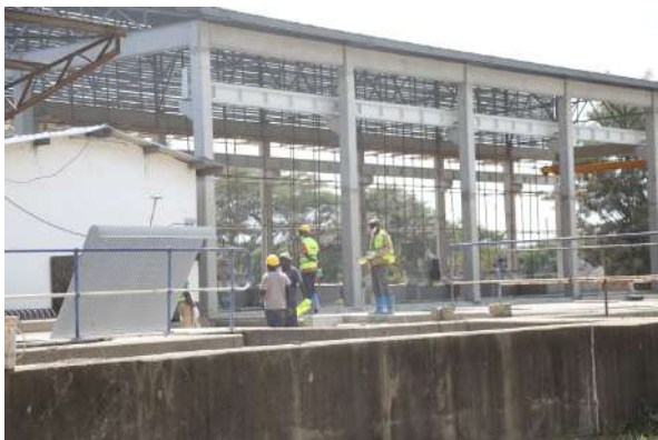
Workers at Dandora Estate Sewage Treatment Works (DESTW) undertaking rehabilitation and expansion of the wastewater facility.
