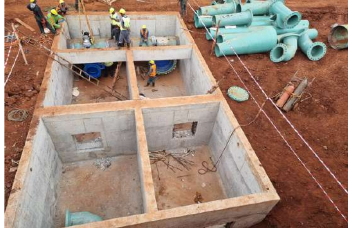
The ongoing inlet works at Gigiri Pumping Station that will receive water from Kegoro Treatment Plant
