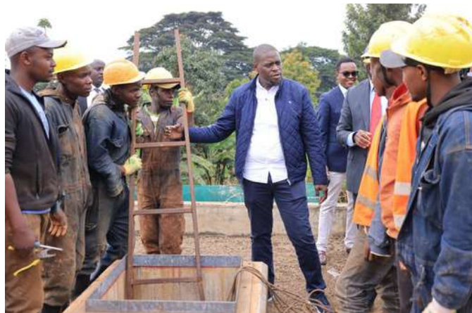
Nairobi City County Governor, H.E Johnson Sakaja, interacting with the workers at Gigiri Pumping Station.
